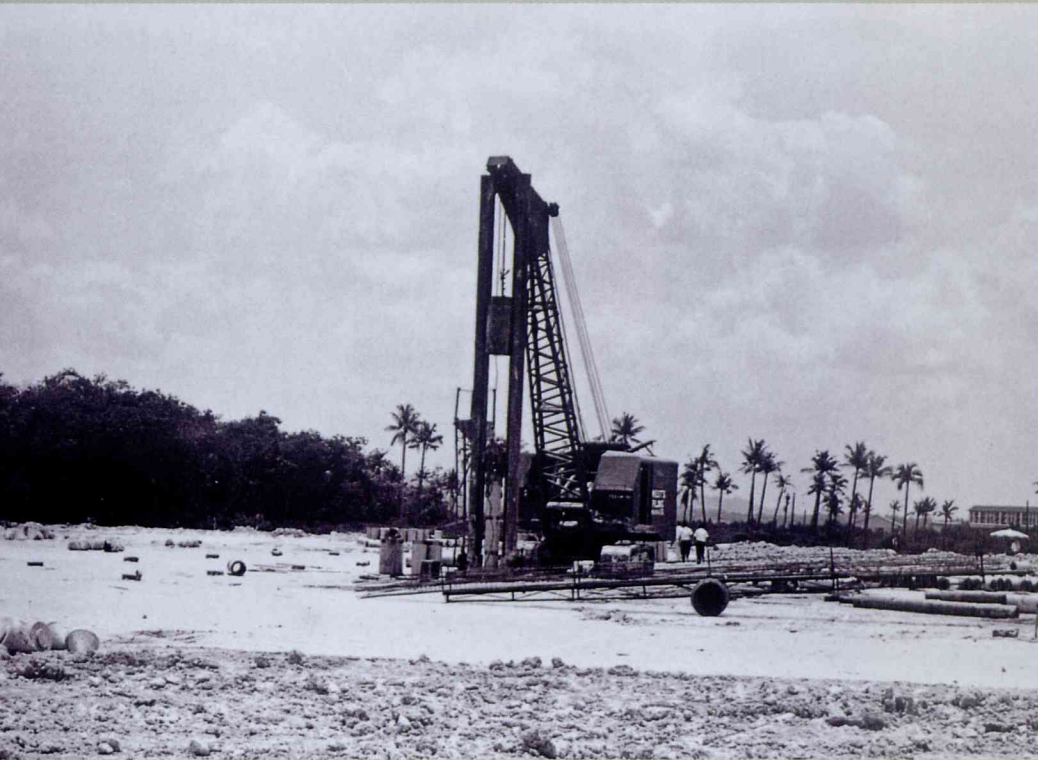
Preparing the ground: construction piling for the Chartered Industries factory at Boon Lay, 1967.
