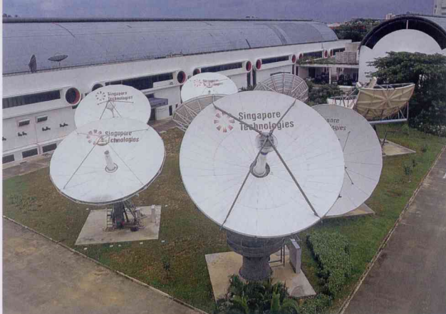
ST Teleport's facilities at Ayer Rajah offer state-of-the-art C-band uplink/downlink to several satellites.
