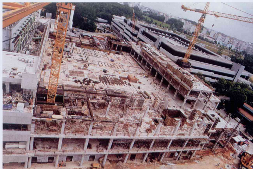
Fab 3 under construction. A semiconductor wafer fabrication plant is called a 'Fab'. CSM's first Fab cost upwards of S$300 million, and was set up in 1988. Fab 2 cost S$1.3 billion and Fab 3, due for completion in late 1997, will cost S$1.8 billion. Other Fabs have been planned, the costs of which are estimated to be at least S$2.5 billion each. Fab 3 will have about 90,000 sq ft of cleanroom space and will produce about 40,000 eight-inch wafers a month.
