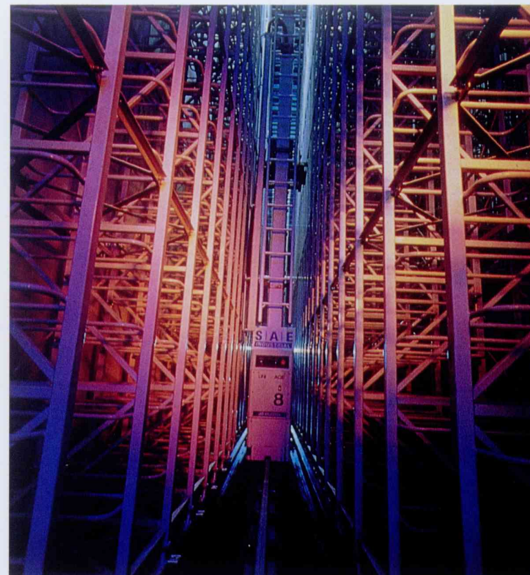
An auto-storage and retrieval system. SAE Industrial Systems does customised design and integration of automated storage and retrieval systems, using automated guided vehicles.
